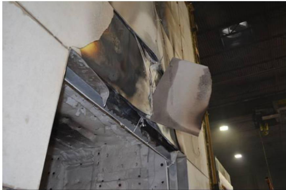
Figure C-15. Close-up of Window Opening immediately after Exposure.
